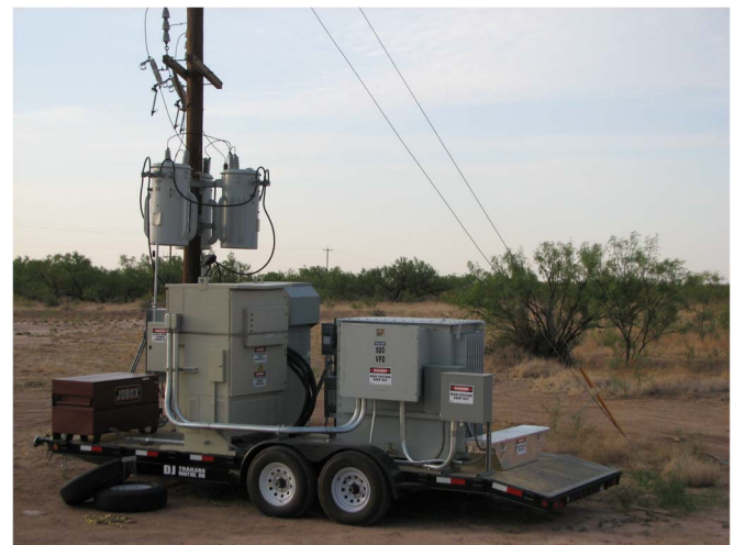
Fig. 12. ESP PMM drive, filter, transformer, and instruments.
